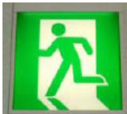
Exit route light
