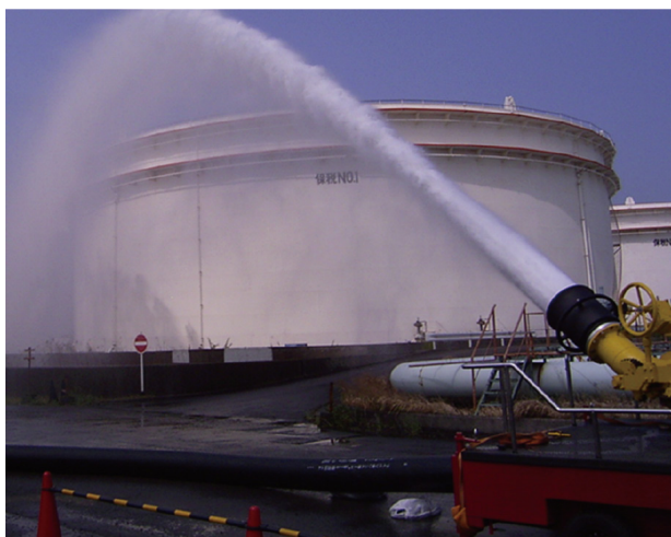
Spraying drills through the use of the high capacity foam system
