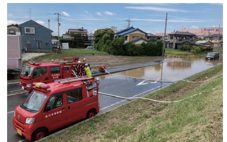
① Drainage Work in Progress by Volunteer Fire Corps (Provided by Yoshikawa City, Saitama Prefecture)
