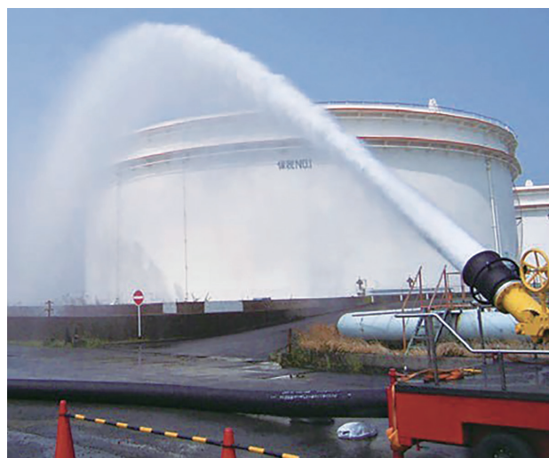
The high capacity foam system
