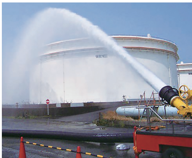
The high capacity foam system
